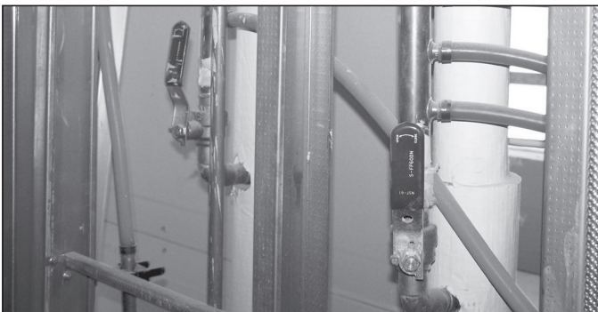
Zurn PEX tubing connected to copper manifolds using copper crimp rings.
