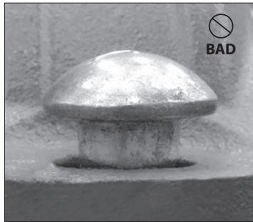
BAD BOLT ENGAGEMENT (OVAL NECK OF BOLT IS NOT SEATED PROPERLY IN THE BOLT HOLE)
