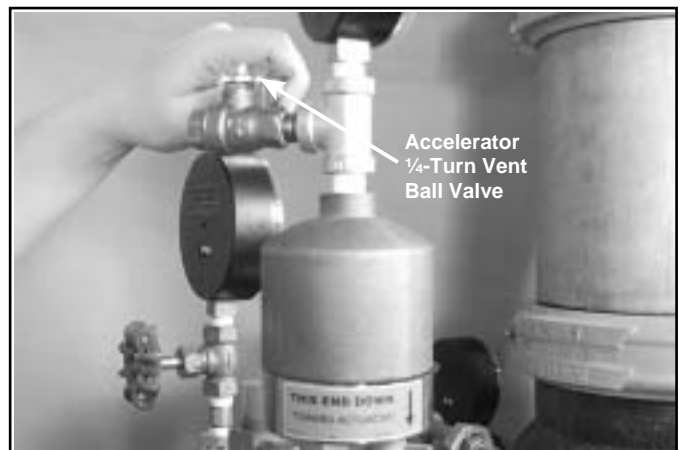
20b. Close ¼-turn vent ball valve. This will set the accelerator.
