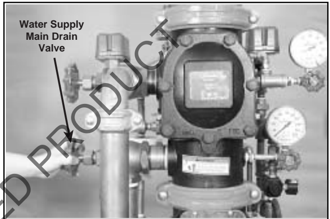
3. Open water supply main drain valve fully to flush water supply of any contaminants.
