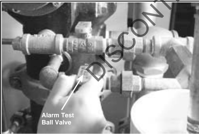
6. Close alarm test ball valve after proper operation of all alarms is verified.
