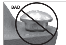
OVAL NECK OF BOLT NOT SEATED PROPERLY
