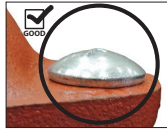
OVAL NECK OF BOLT SEATED PROPERLY
