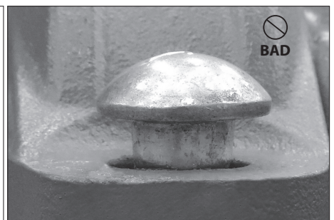
BAD BOLT ENGAGEMENT (OVAL NECK IS NOT SEATED PROPERLY IN THE BOLT HOLE)
