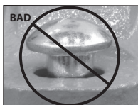
OVAL NECK OF BOLT NOT SEATED PROPERLY
