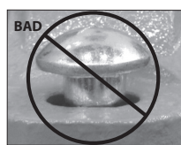
OVAL NECK OF BOLT NOT SEATED PROPERLY
