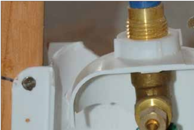
Cheap Materials. Brittle and thin styrene boxes are easily damaged by job site abuse.
