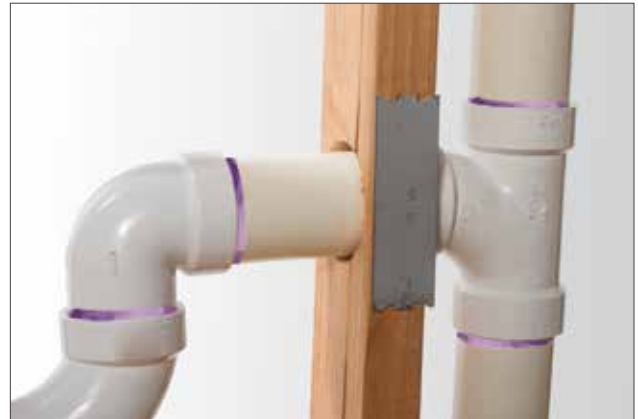
Stud Protection Needed. Drain line in second stud bay needs added protection and reinforcement.
