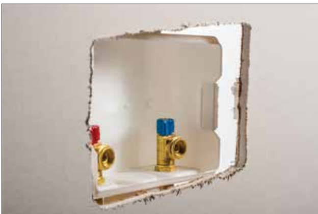
Brackets Are Easily Cut. Rotozip drywall cutters often cut right through thin styrene brackets leaving the plumbing as the only support.
