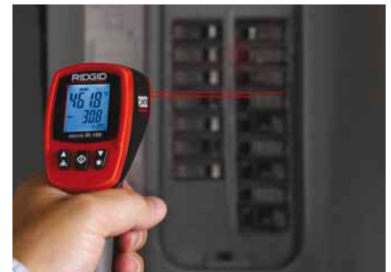
Check fuse or circuit breaker overheating, which could be caused by overloaded circuits
