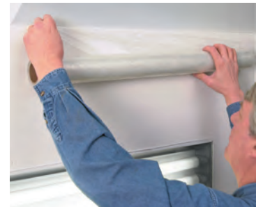
Beginning at one end of the wall, tack down a 2"-3" starter edge at the ceiling break.
