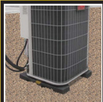
Air Conditioning Support
