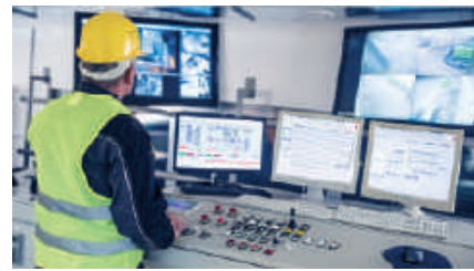
Remote Control Room
