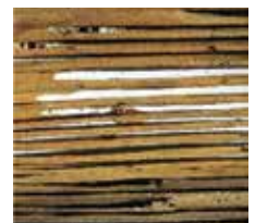
CARPENTER ANT DAMAGE
