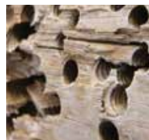
CARPENTER BEE DAMAGE
