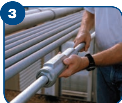
3 Thread the next length of conduit into the other end of the fitting and tighten. You're done!
