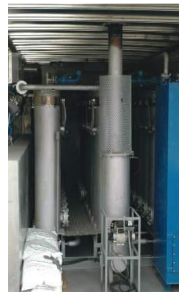
Plant Filtration Columns
