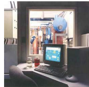
Plant Control Room
