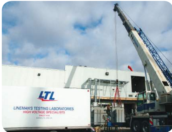
Substation/Engineering Services & Equipment Supply
