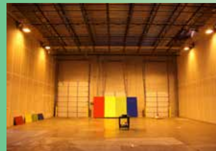
250W HPS Floodlight (280W Actual)
