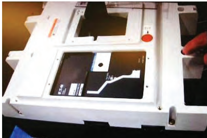
Figure 1. Trip Unit Clear Cover Removed.
