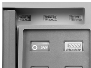
Accessory Viewing Windows Visibly Confirm the Breaker Shunt Trip, Spring Release, and UVR Installation and Their Control Voltage Rating
