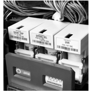
Shunt Trip, Spring Release and Undervoltage Release Device Installed on Accessory Deck
