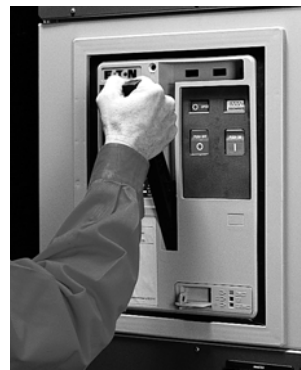
Through-the-Door Design for Human Interface with the Breaker Compartment Door Closed, for Example, Manually Charging the Stored Energy Springs
