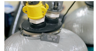
General Mechanical Identification
