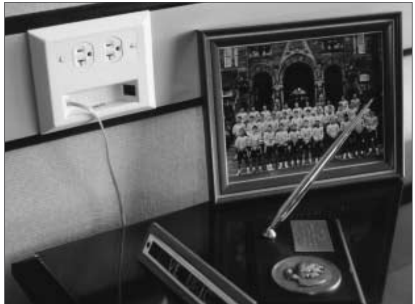
Access 5000 Raceway installed at chair rail height.
