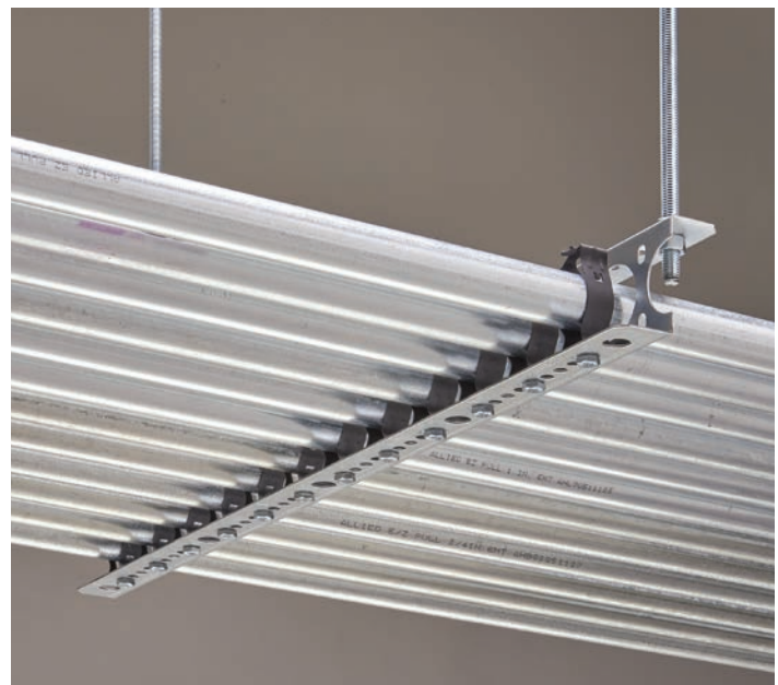
Conduit trapeze support with Guide-Rite™ fasteners
