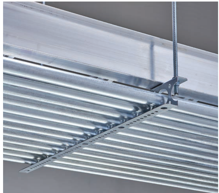
Conduit trapeze support with cable tray
