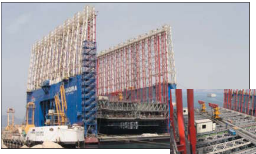
▼ PLC-controlled hydraulic movement: Enerpac stage -lift systems lift and lower the umbrella deck on the world's largest concrete block builder with 0,01 mm accuracy, provided by 30 hydraulic climbing units in an integrated hydraulic system.
