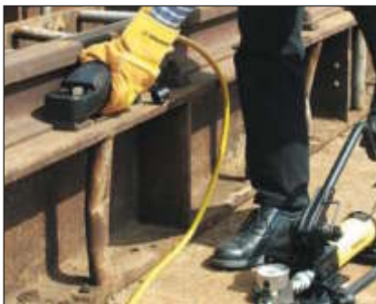
◀ Easily removing rusty nuts during railroad construction is just one of many application examples for the Enerpac Nut Splitter.
