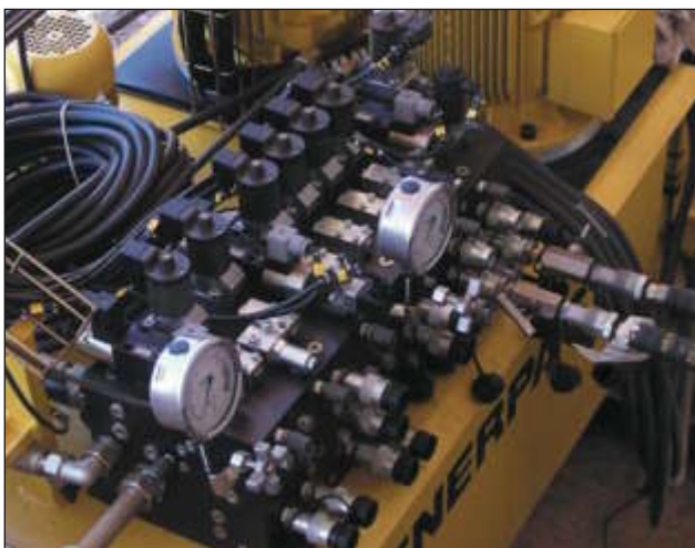
◀ A typical multi-cylinder control set-up using solenoid directional control valves.
