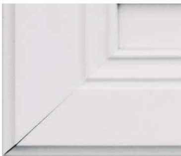
separation of door corner
