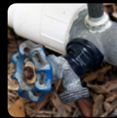
Repairs loose or leaky plumbing
