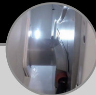
No Flex Pipe! No Dryer Fires!
