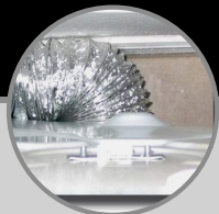
Bulky, Constricted Flex Pipe
