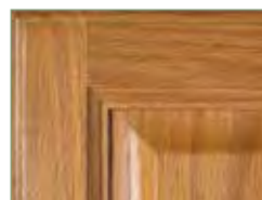
Telegraphing is the effect of the grain showing through the stain. Open or coarse wood grains, like oak, will "telegraph" more than closed or finer wood grains.
