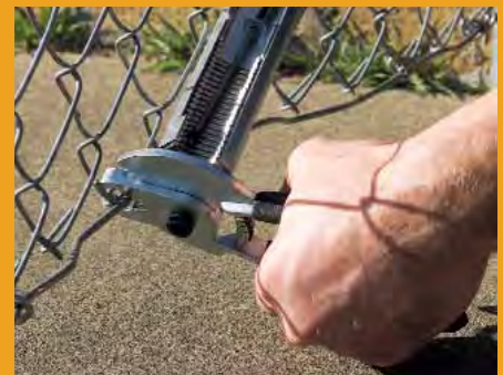
HFP9 Attaching tensioning wire to chainlink fence with 9 gauge aluminum hog rings
