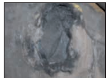
Melted or Charred areas
